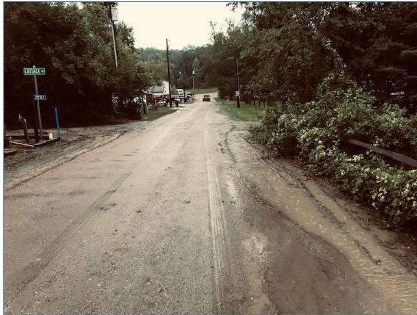
Photograph 4 is facing east at the intersection of Cottage Drive and Webster Boulevard. This is where the ditches are not functioning correctly (Dan Pearson -2019).
