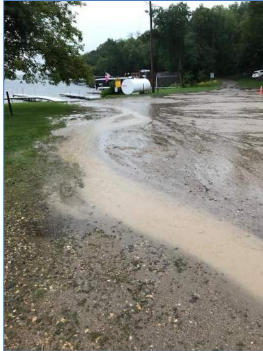
Photograph 14 is facing northeast from the west building of the lodge. In the background of the photograph near the dock is the proposed location of the grass pavement system. This system will filter the surface water through the grass and allow water to soak into a course rock subgrade (Dan Pearson - 2019).
