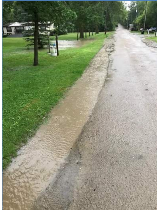
Photograph 5 is facing west on Webster Boulevard from near the intersection of Huggett Lane. Water can be seen in the secondary ditch. This is the area where the maintenance needs to be complete to remove the secondary ditch and re-establish the ditch. (Dan Pearson -2019).
