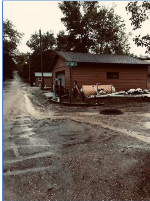
Photograph 2 is facing west at the intersection of Webster Boulevard and Cottage Drive. This is an example where a secondary ditch needs modification. (Dan Pearson - 2019)
