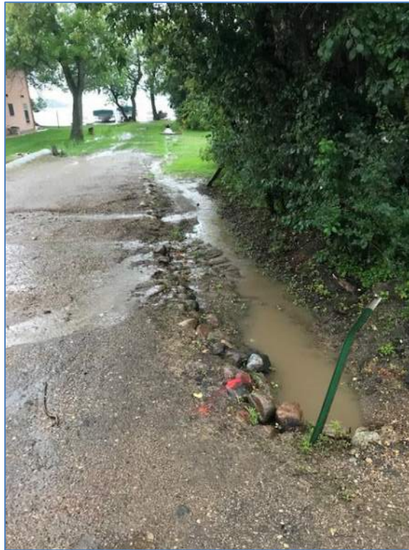
Photograph 11 is looking north down Cottage Drive from Webster Boulevard. This photograph is an example of ditch re-establishment and improving the surface using a grass pavement system (Dan Pearson - 2019).
