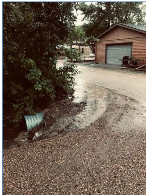
Photograph 3 is looking at the culvert in the southwest corner of the intersection of Webster Boulevard and Cottage Drive. The water from the west is not correctly entering the culvert. Work at this location consists of re-establishing the ditch from the west. (Dan Pearson -2019).
